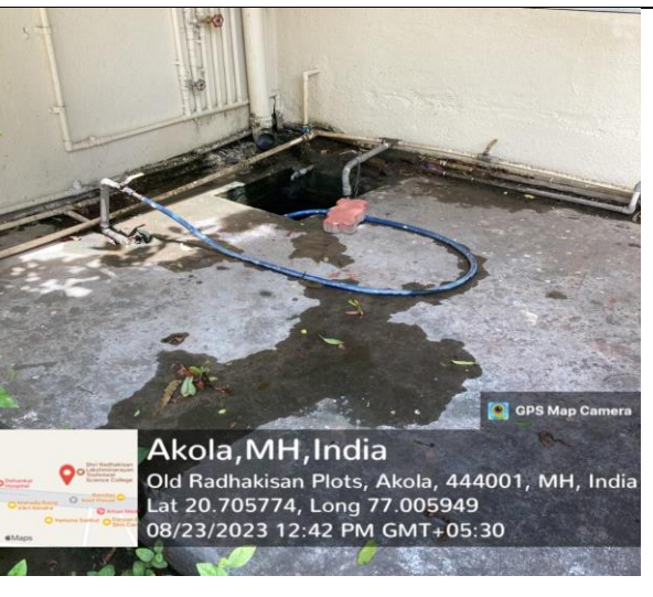
Underground tank having capacity 15000 liters
