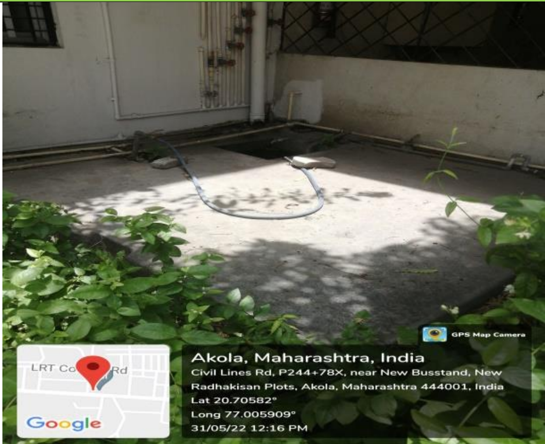
Underground tank in campus having capacity of 15,000 litres
