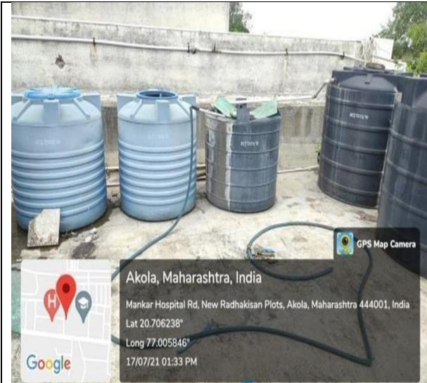
Sample tanks on the roof of wing D out of 31
