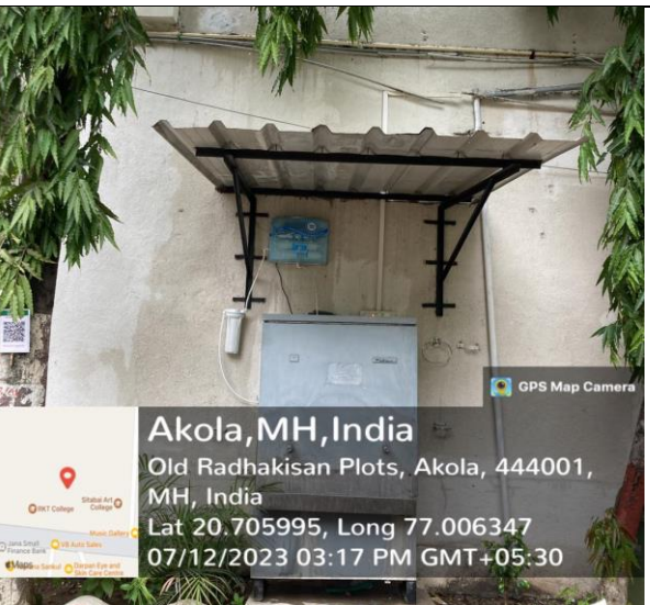
7 water coolers to provide cold water
