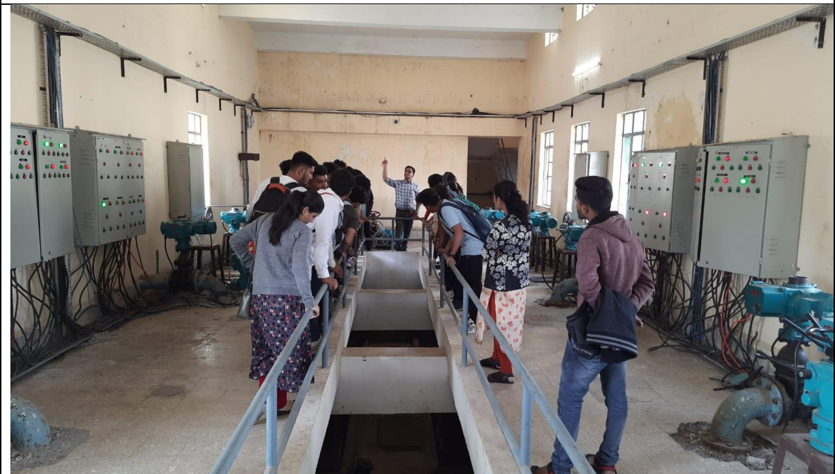
Control Unit Of Sedimentation Tank
