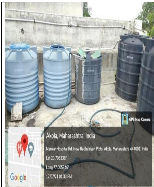
Sample tanks on the roof of wing D out of 31 tanks
