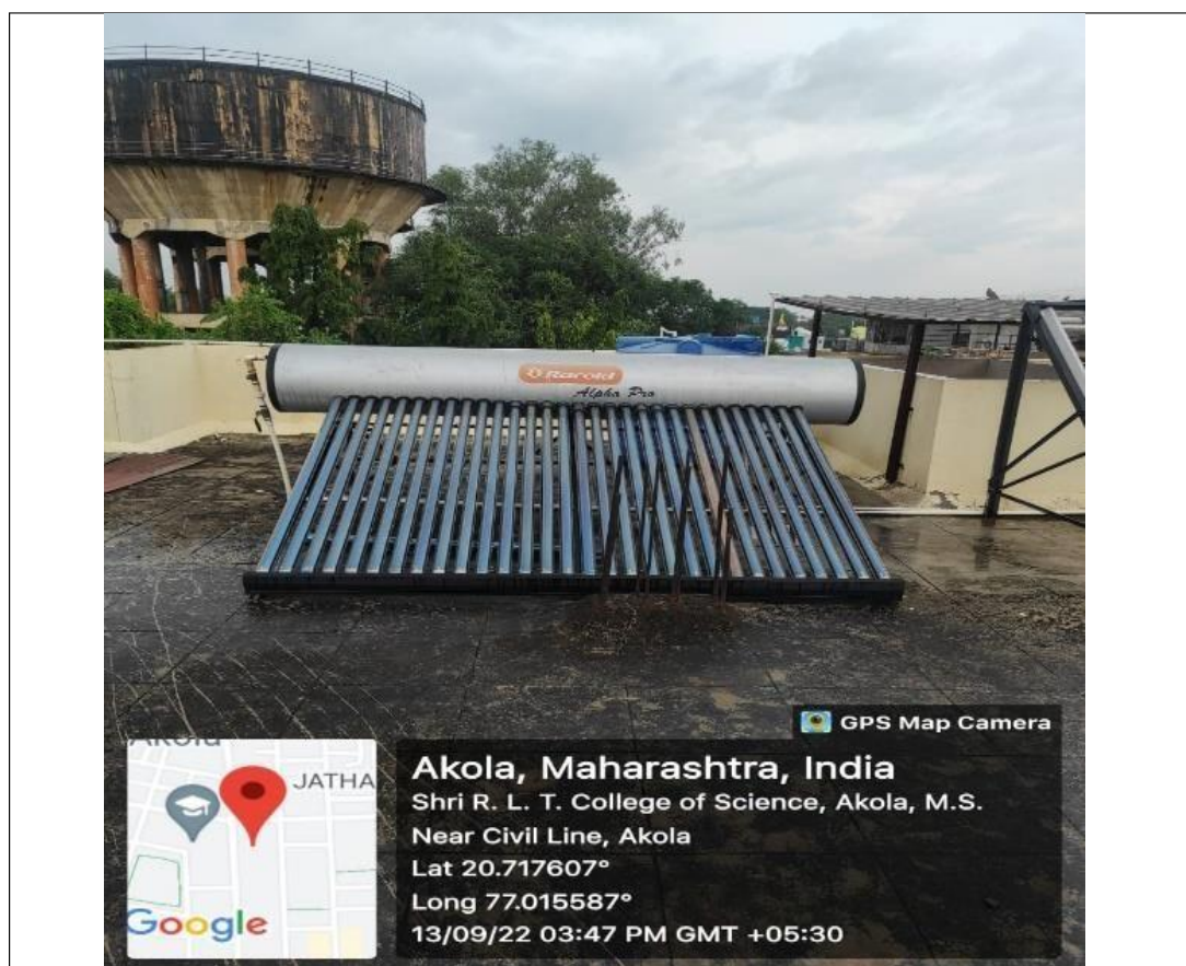
Solar water heater in girl's hostel
