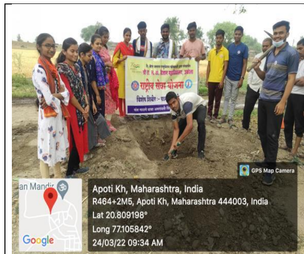
NSS volunteers were prepared 4 soak pits at different 4 places in adopted village.
