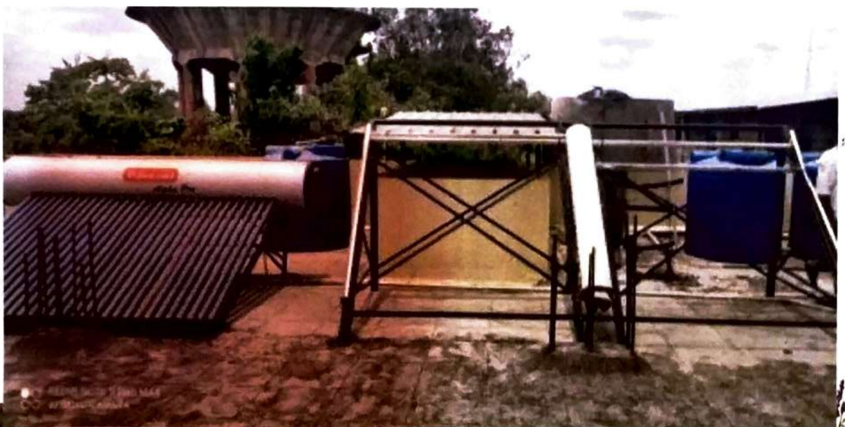
Solar water installed at Girls Hostel reduced electrical energy consumption at a great extent.
