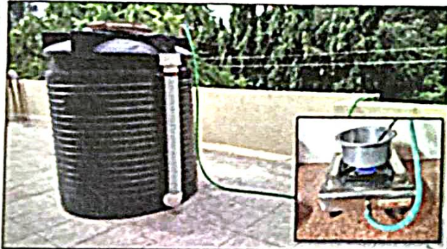
Biogas Plant in Girl's Hostel
