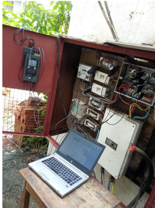
Figure 18 MSEDCL Meter Panel
