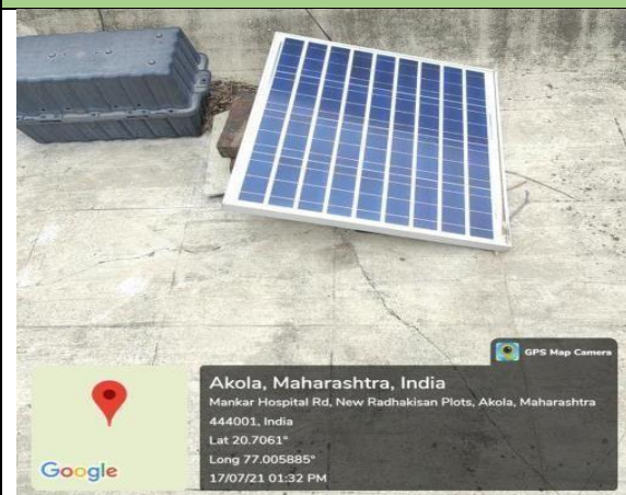
Solar panels of solar based LED lights
