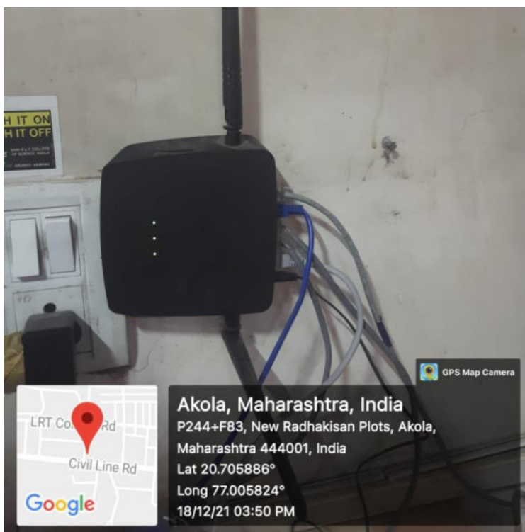
Office Airtel Router (100 mbps)
