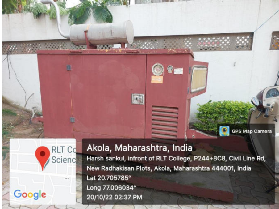
Power Generator 10 KVA
