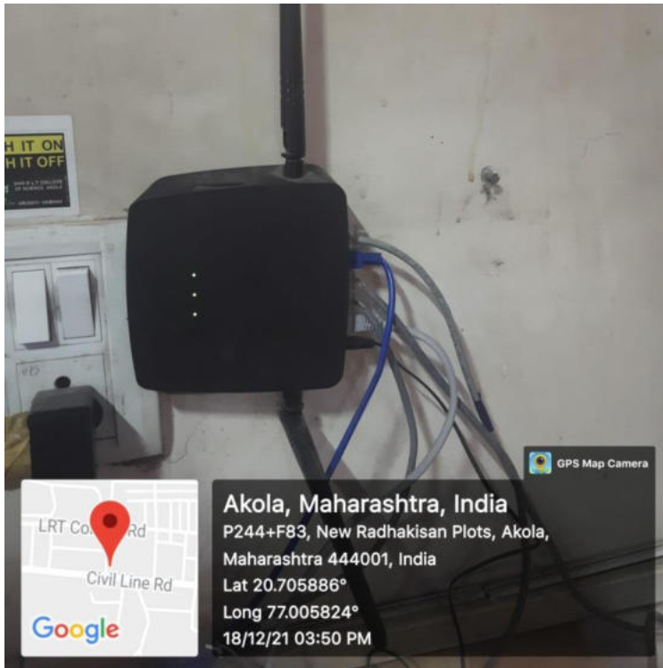
Office Airtel Router (100 mbps)
