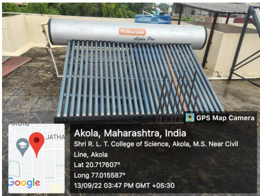
Solar Water Heater (Hostel)
