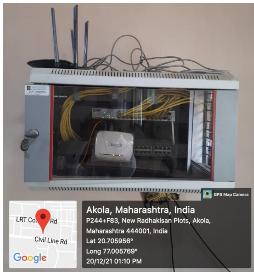
Computer Science Lab Fiber Optic Connection Router BSNL (100 mbps)
