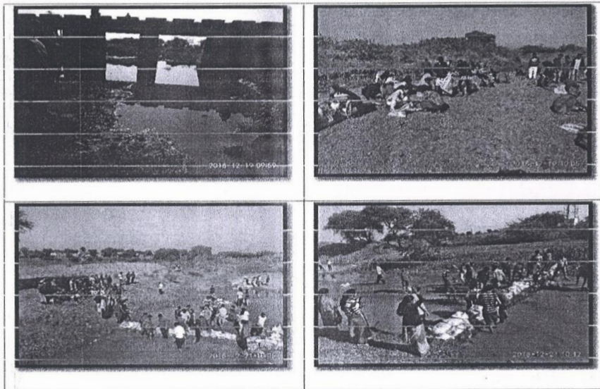
Construction of Vanarai bandhara on the Lonar canal of the adopted village Aapoti (Kd)
